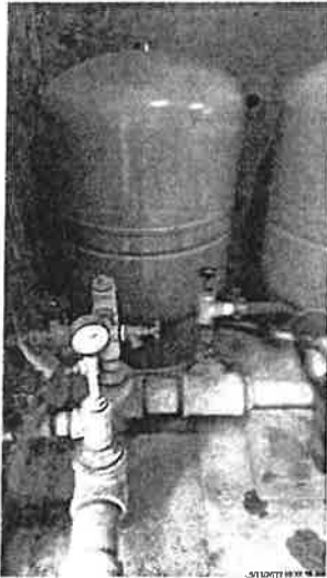
Pressure release-valve at BPS
