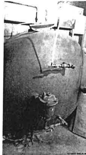
Hydropneumatic tank with pumphouse
