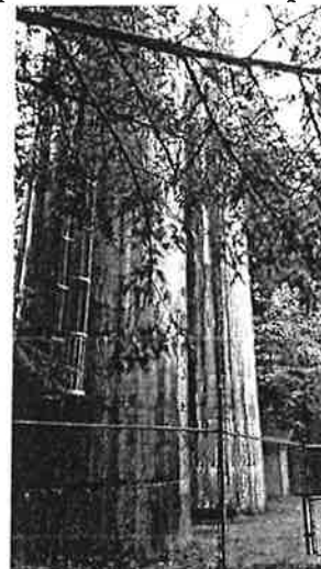
Finished water reservoirs
