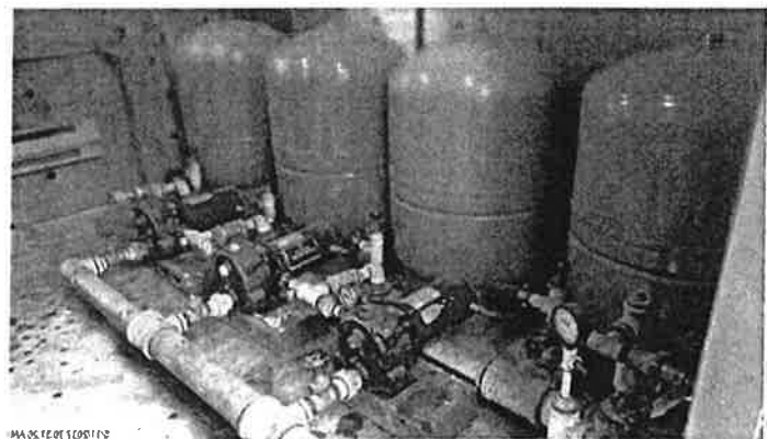
Incline Drive Booster pump station
