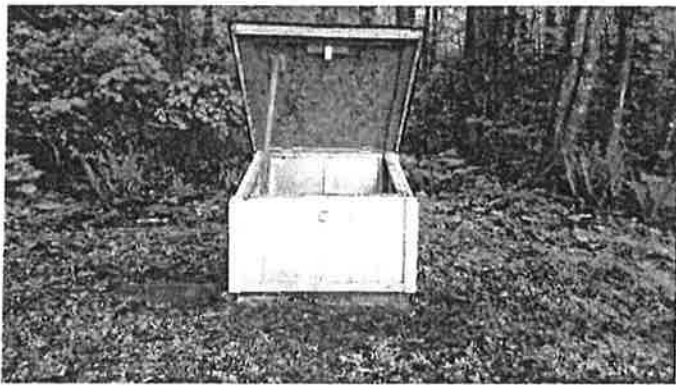
Well #5 enclosure with broken lock hasp
