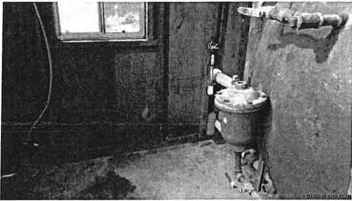
Oil-less air compressor in pumphouse
